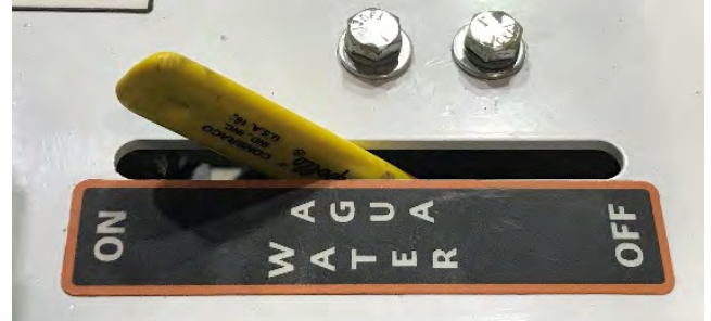
Water Valve - ON
