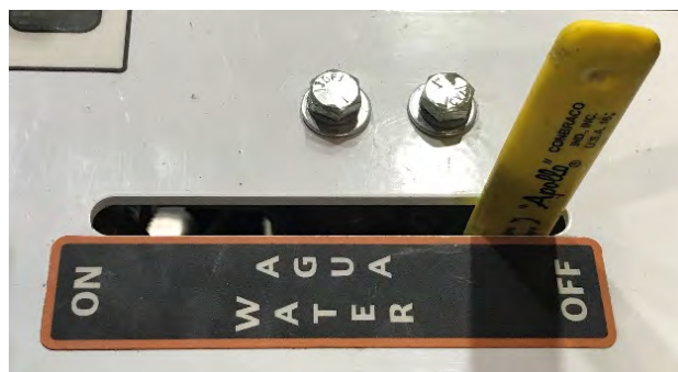
Water Valve - OFF
