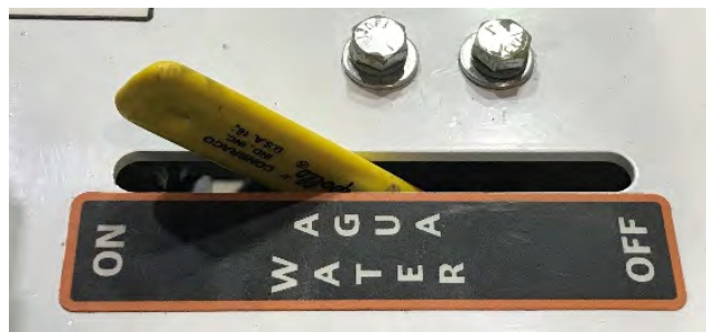
Water Valve - ON
