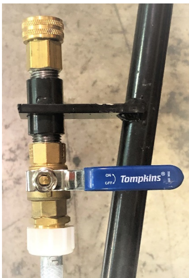
Water Supply Valve
