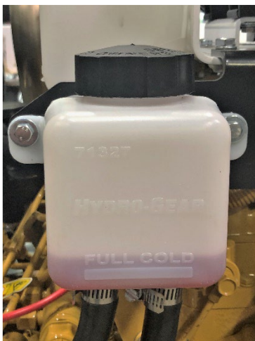
Hydro Pump Reservoir Tank
