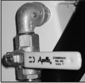
Figure 26: Right Water Valve
