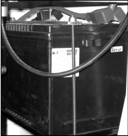
Figure 67: Battery and Brace
