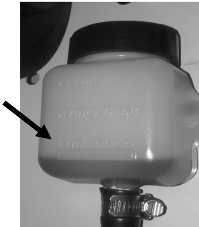
Figure 81 Expansion Tank Cold Line
