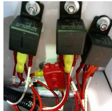
Figure 69: Circuit Breaker and Relays
