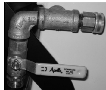
Figure 25: Left Water Valve
