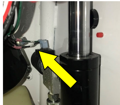
Solenoid Block Wires
